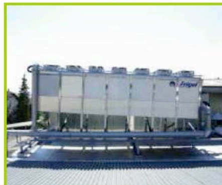
New Cooling System
